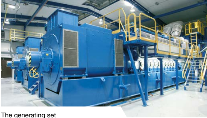
The generating set
